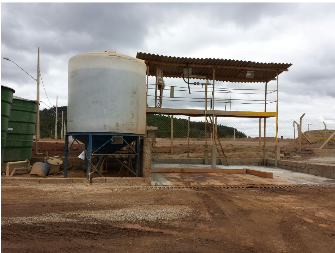
Figura 3 – Central de concreto
